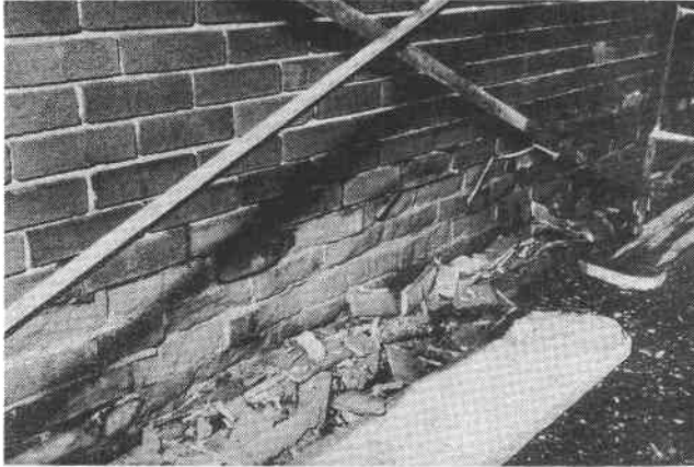
Figure 4. Laminar break-up of masonry units which were covered by a metal flashing.
